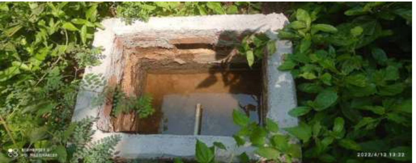
Fig 4: Pipeline for Rainwater Harvesting
